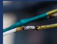
Defective or inadequate insulation
