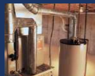
Water Heater Issue
