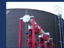
Water tanks pressure & supply
