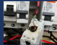
Loose Connections / parts
