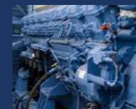
Power supply to fire fighting system
