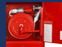
Fire Safety Equipment
