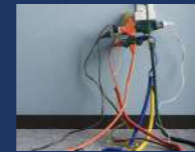
Overloading or inadequate capacity
